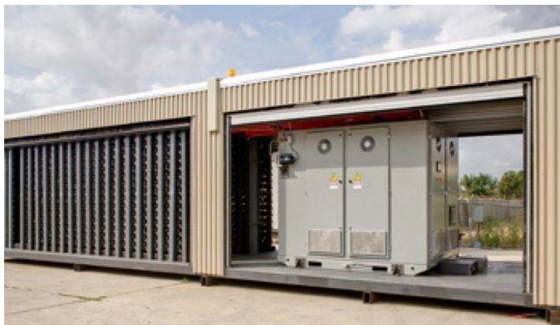
Figure 3 Example of an ESS that caught fire on the Kahuhu windfarm
