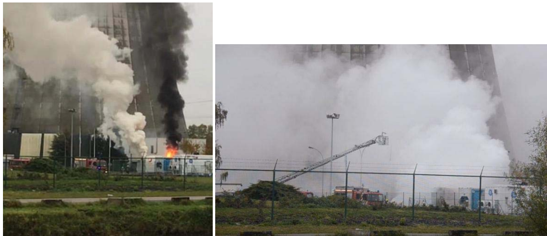
Figure 2 Fire of a 1MW battery container in Drogenbos (Belgium)
